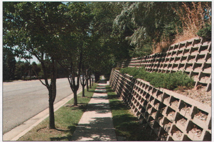
Looking east on the north side of Parleys Way. The retaining wall on the right holds up the existing Kmart parking lot.
